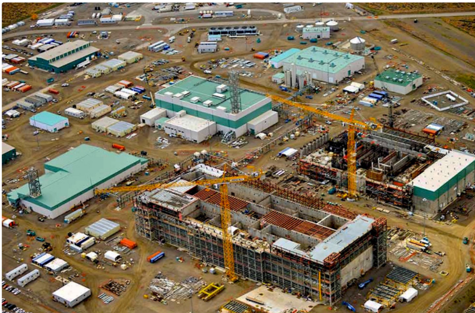
The Waste Treatment and Immobilization Plant (WTP) being designed and constructed by Bechtel National for the US Department of Energy at Hanford in Washington State, USA. When complete, the WTP will be the world's largest radioactive waste treatment plant
